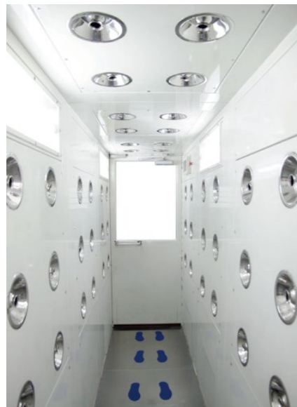
Air shower for workers
